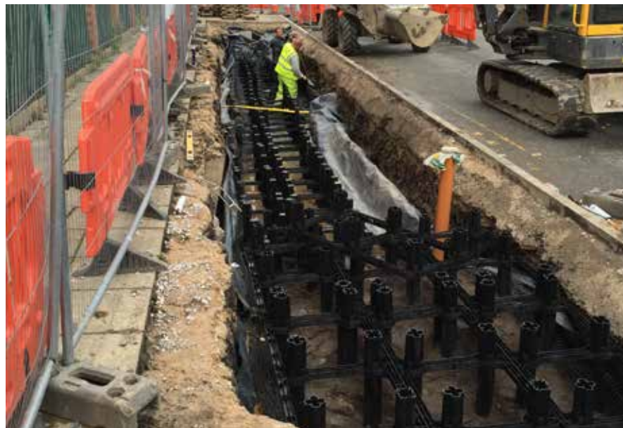
DeepRoot SilvaCells used for retrofitting tree planting in Howard Street Salford, where three years of monitoring rainfall events by the University of Manchester showed an average reduction of 85% in peak and 80% in volume, with a peak-to-peak delay of 118 minutes. © DeepRoot
