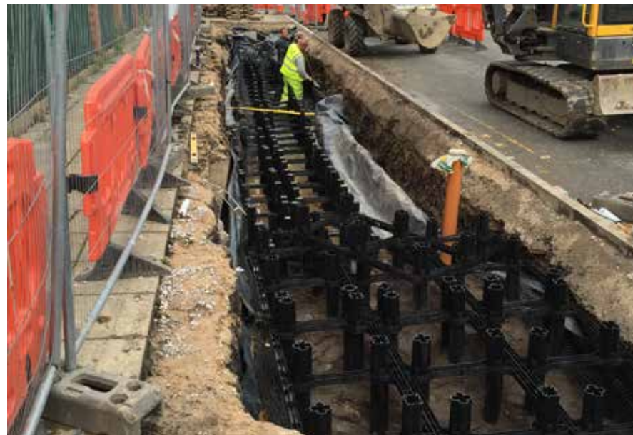
DeepRoot SilvaCells used for retrofitting tree planting in Howard Street Salford, where three years of monitoring rainfall events by the University of Manchester showed an average reduction of 85% in peak and 80% in volume, with a peak-to-peak delay of 118 minutes. © DeepRoot
