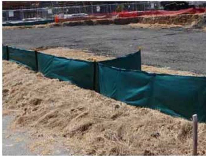
Geotextile silt fence combined with straw on a housing site in New Zealand
