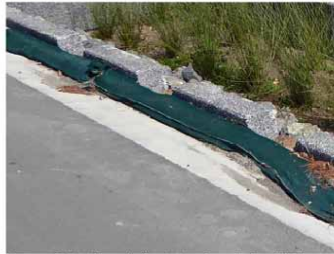
Temporary Geotextile sand roll protects a rain garden from siltation near a construction site in Hobsonville, New Zealand
