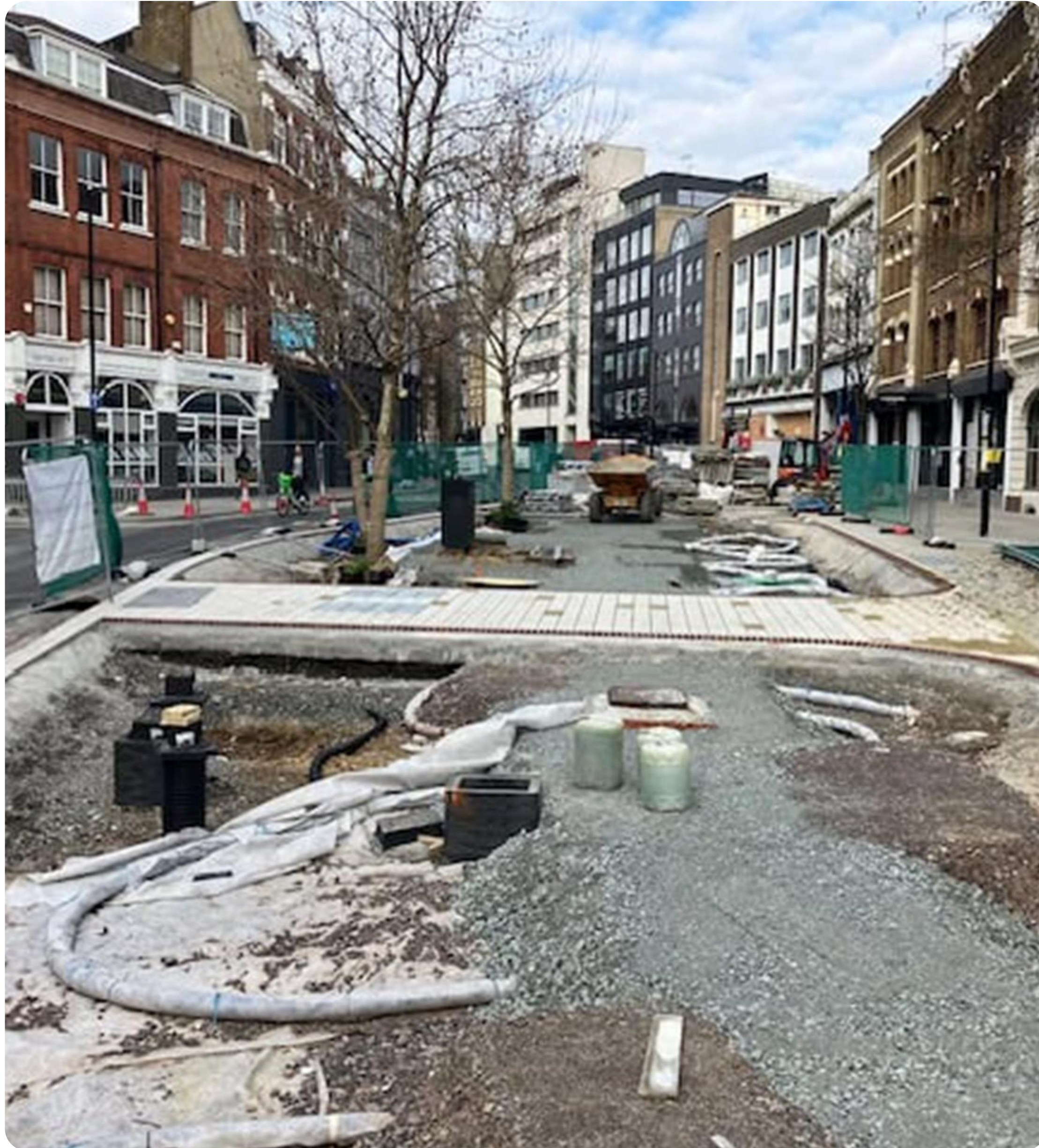
St John Street – London Borough of Islington, during SuDS retrofit works Image courtesy of Meristem Design
