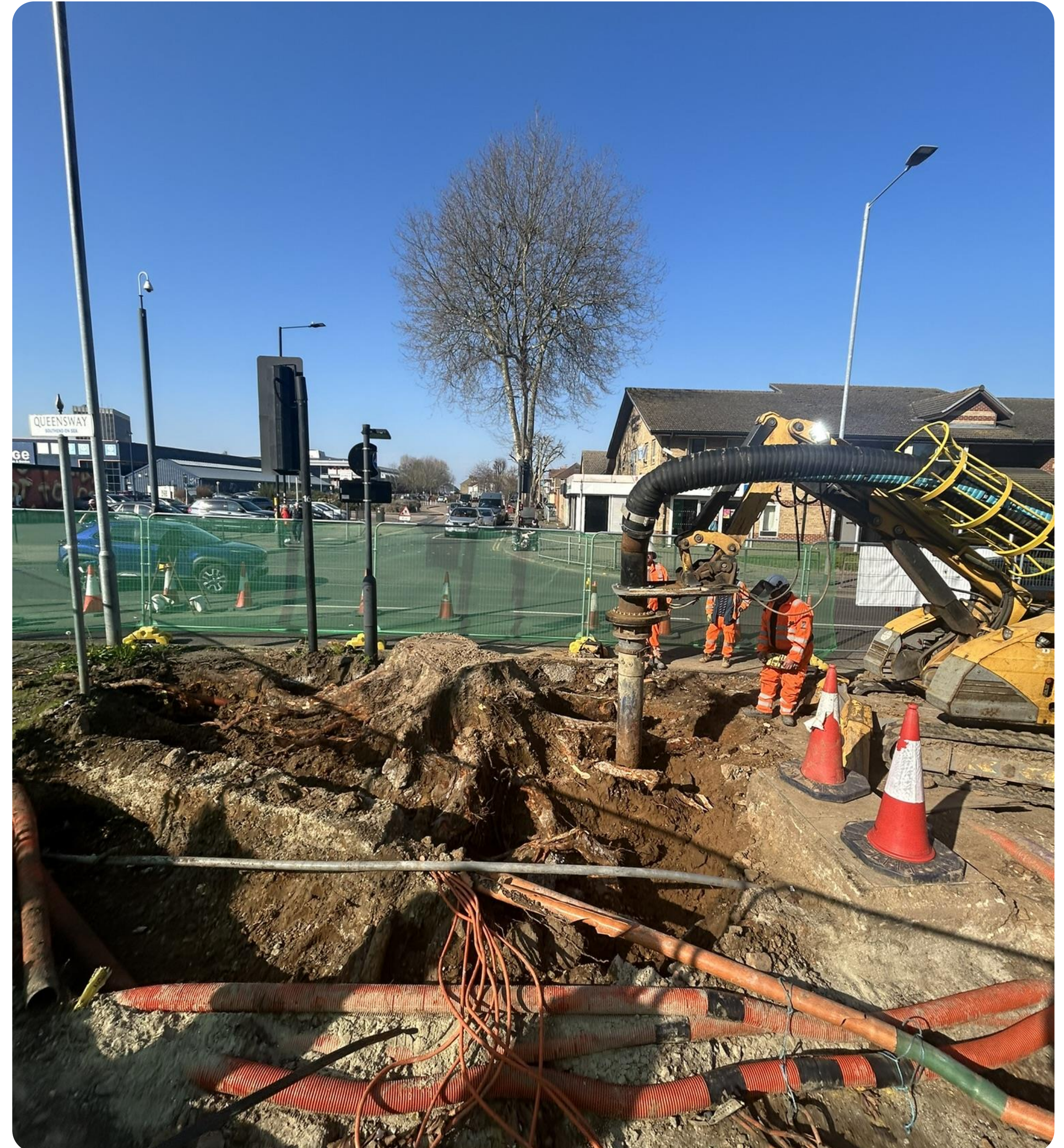
Vacuum Excavation Around Felled Tree Stump & Live Utilities Image courtesy of Civic
