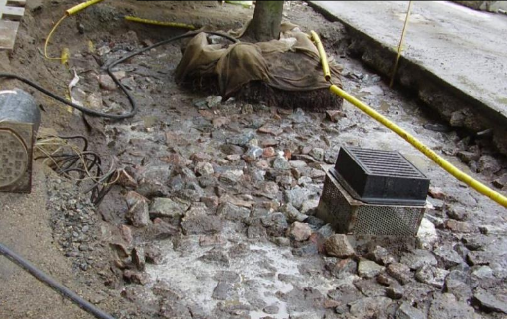
Ventilation chamber and inlet of surface water
