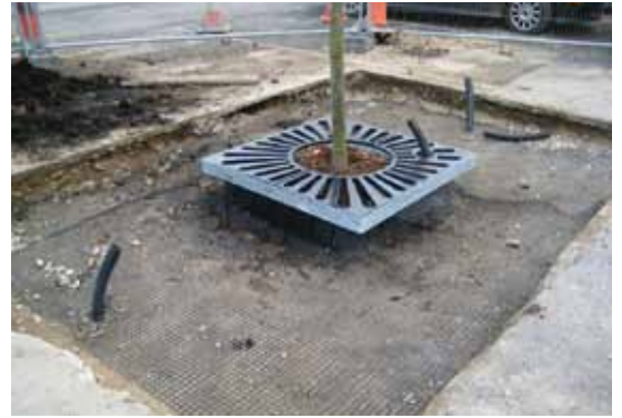
Tree planted within root deflector; grill in place ready for surface reinstatement
