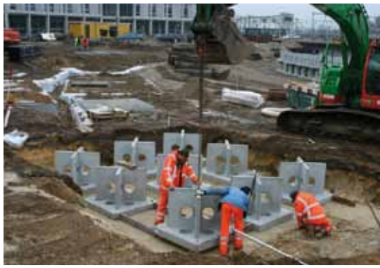
Positioning concrete crates on prepared island base at Apeldoorn station square (see Case study 22)
