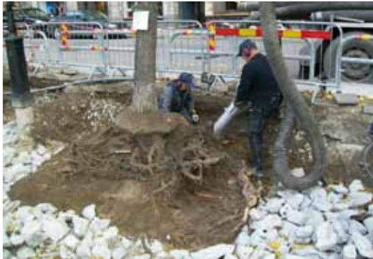
Some roots have been pruned. Excavation and soil clearing near the root ball is carefully conducted with non-invasive tool
