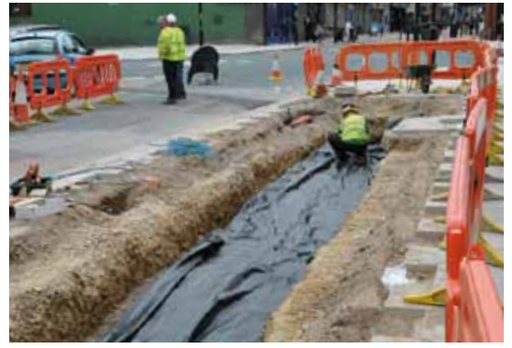
Root barrier lining
