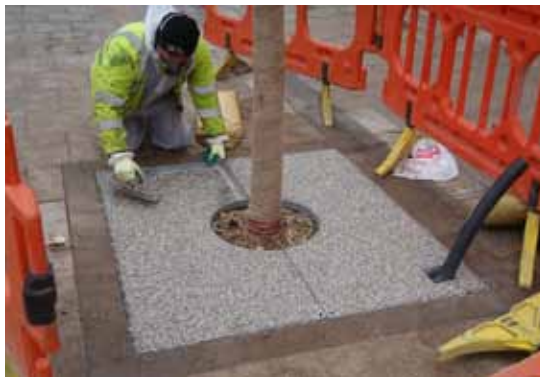
Grate with watering inlet and resin-bound infill and watering/aeration inlet on Ocean Road (see Case study 2). Image: South Tyneside Council
