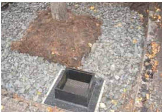
The aeration layer of smaller dry rock has been placed over the skeleton soil. It includes an aeration well, to be capped with a grate sitting flush with the paving
