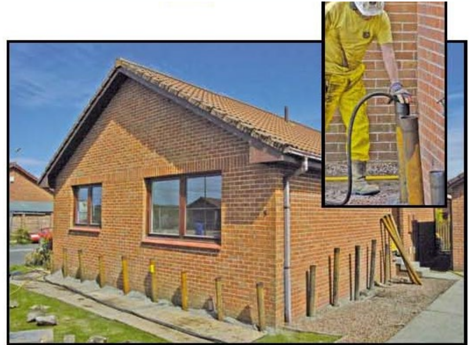
External Angle Piles - Ready for driving (Inset - External Angle Piles - Being driven to suitable bearing stratum)
