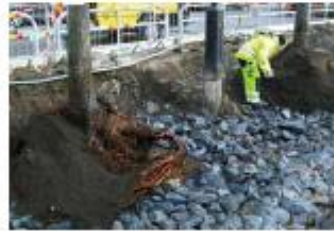
High quality soil is applied around the pruned/dead root balls. Notice the root deformations caused by deep concrete casing used in the earlier planting hole design.
