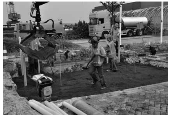
Filling with 100% recycled sand-based structural soil in 30 cm layers, well compacted with a vibrating (wacker) plate.
