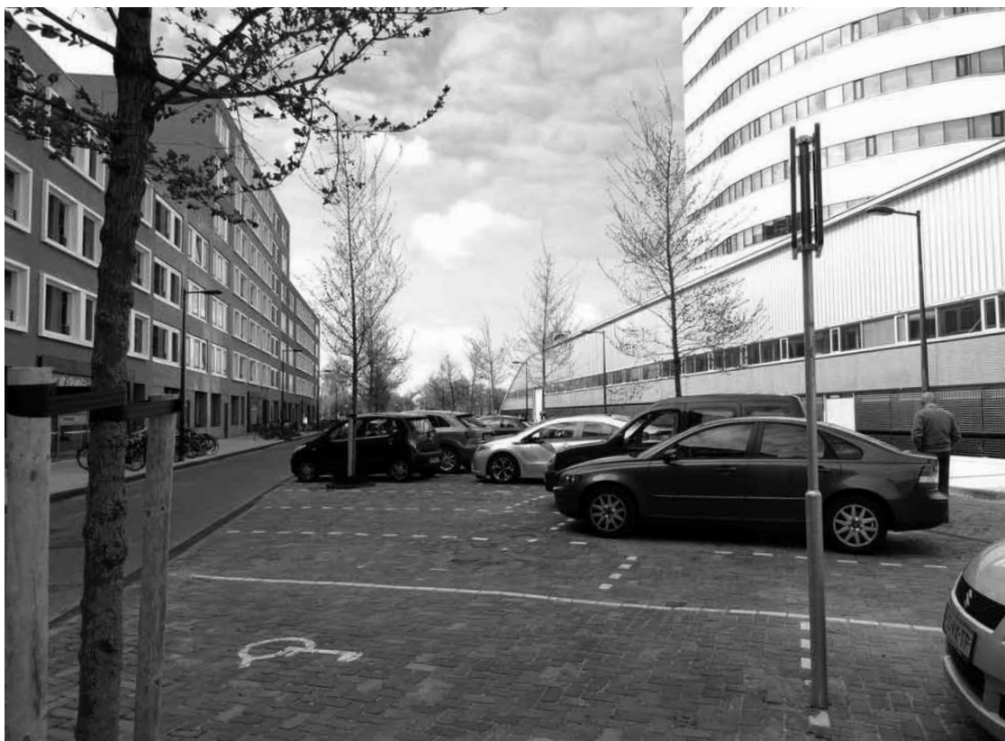
Newly installed permeable paving laid over a raft system (Permavoid Sandwich Construction) in Amsterdam, The Netherlands. Image: Jeremy Barrell
