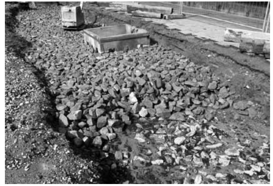
Soil has been flushed into the first layer of compacted large stones. A second layer of large stones is being applied.
