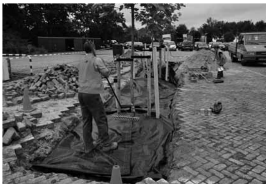
Trees planted, geotextile in place to prepare the foundation for the concrete block pavers.
