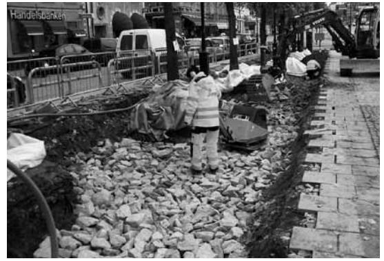
Large stones for the skeleton soil layer are being positioned and compacted in the newly created continuous trench.
