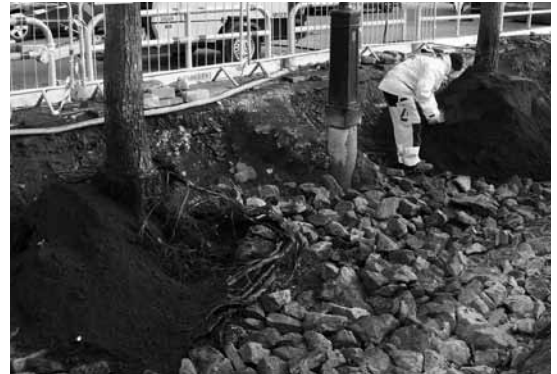
High quality soil is applied around the pruned/cleared root balls. Notice the root deformations caused by deep concrete casing used in the earlier planting hole design.
