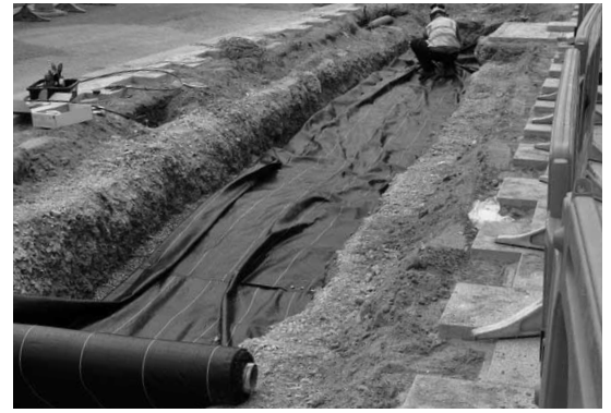
Root barrier lining.
