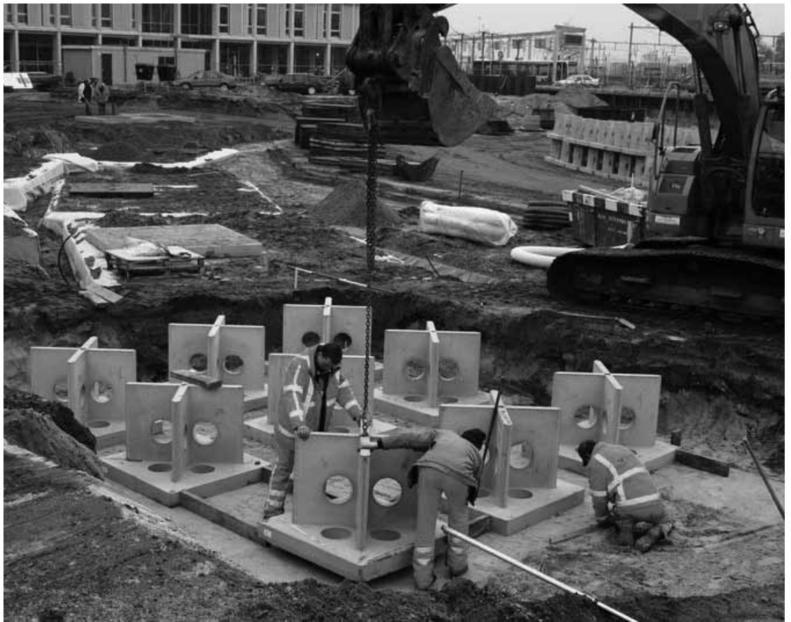
Positioning concrete crates on prepared island base at Apeldoorn station square (see Case study 24, p127).
