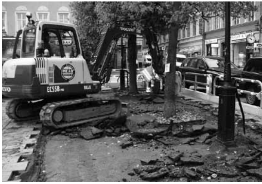
Excavations start on Kornhamnstorg a public square in Stockholm's old town where lime trees show early sign of decline.
