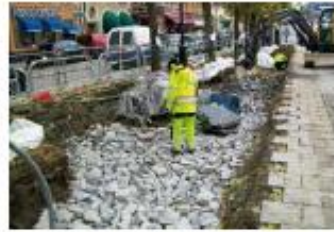
Large stones for the skeleton soil layer are being positioned and compacted in the newly created continuous trench.
